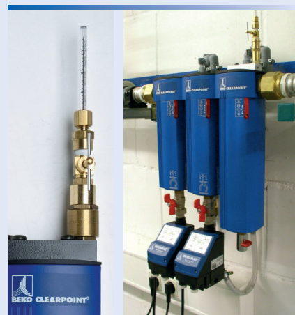
CLEARPOINT® prefilter type F and S with BEKOMAT® 20 FM condensate drain, CLEARPOINT® V activated carbon adsorber with oil check indicator
